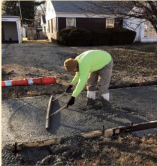
Approximately 3,714 linear feet of new sidewalk were constructed in February 2020 in the Delaware neighborhood, thanks to the City's Neighborhood Works capital improvement grant program.
