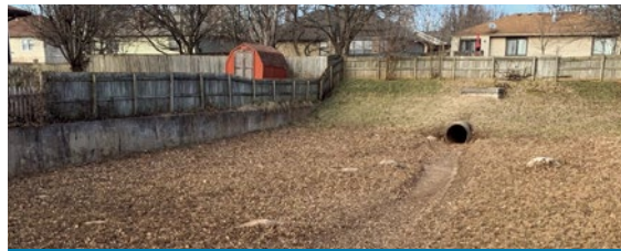
Detention basin at Seminole Street and Nettleton Avenue.
